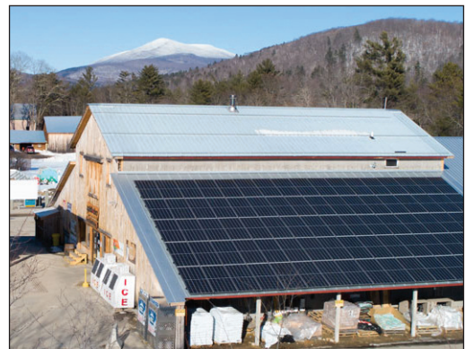
NH Solar Shares' second community solar PV array is located on the roof of Appleknockers General Store in Warren.
